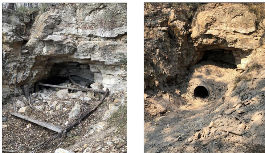
Photo 1 Rock Debris Pile “Before: and Inserted Culvert “After” at the Entrance of the Mine Adit
