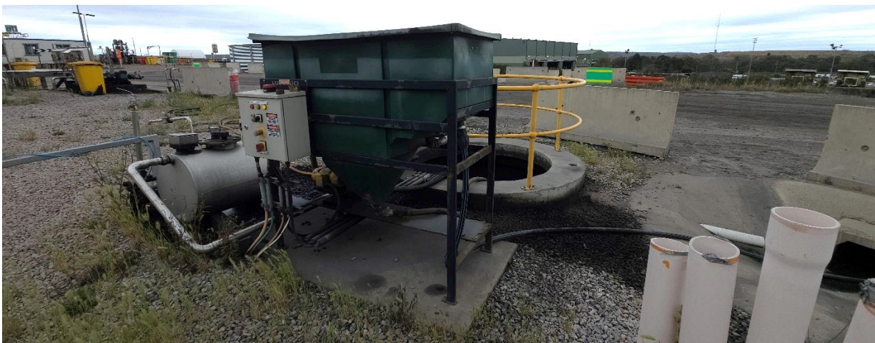
Plate 8 Oily water separator at fuel storage and refuelling area near workshop
