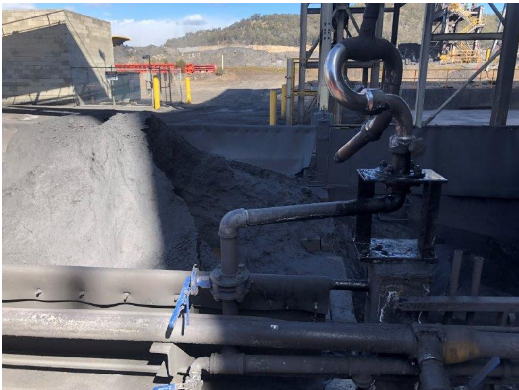
Plate 10 – Magnesium storage area with dust suppression systems in place
