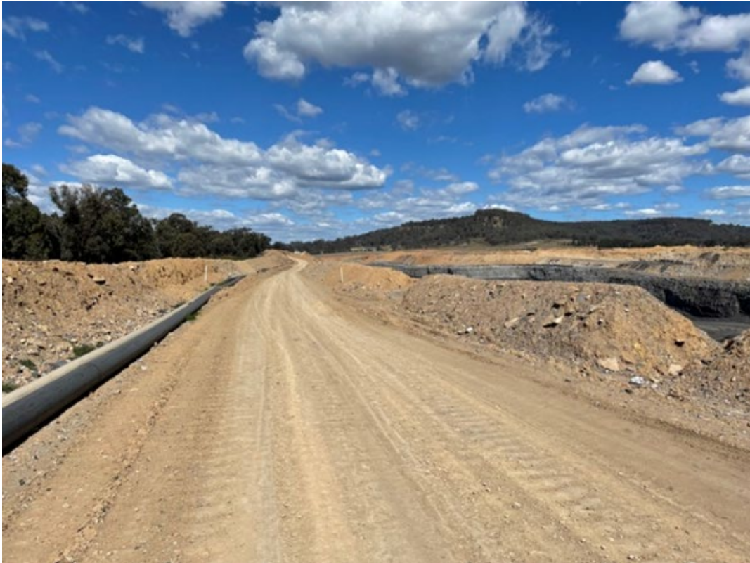
Plate 43 – Example of Water Management on Downslope Perimeter to prevent offsite discharge (pit 8)
