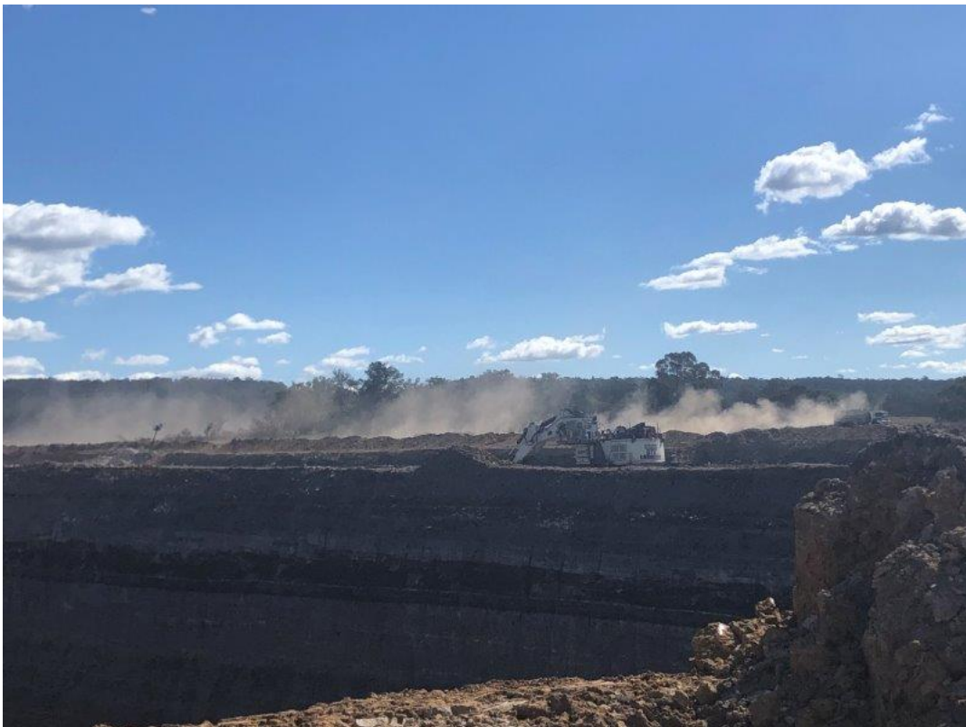
Plate 26 – Dust production along top of pit adjacent Ulan-Wollar Road near Pit 6
