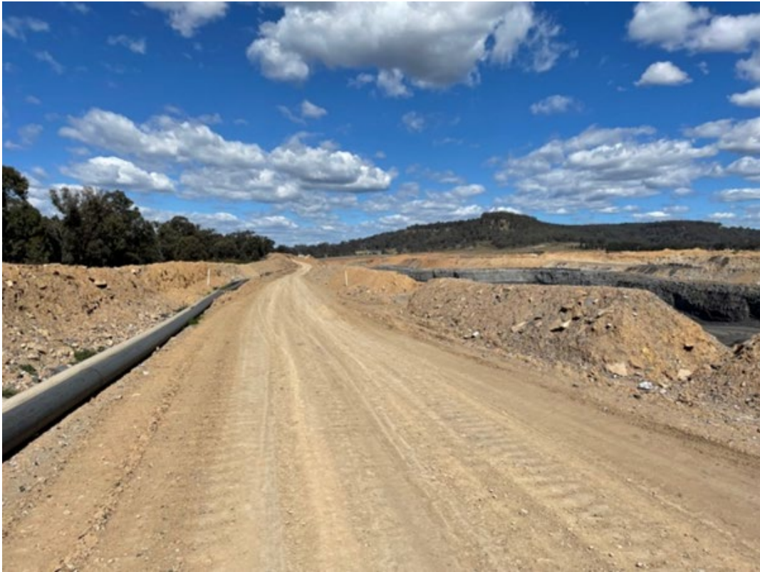
Plate 43 – Example of Water Management on Downslope Perimeter to prevent offsite discharge (pit 8)
