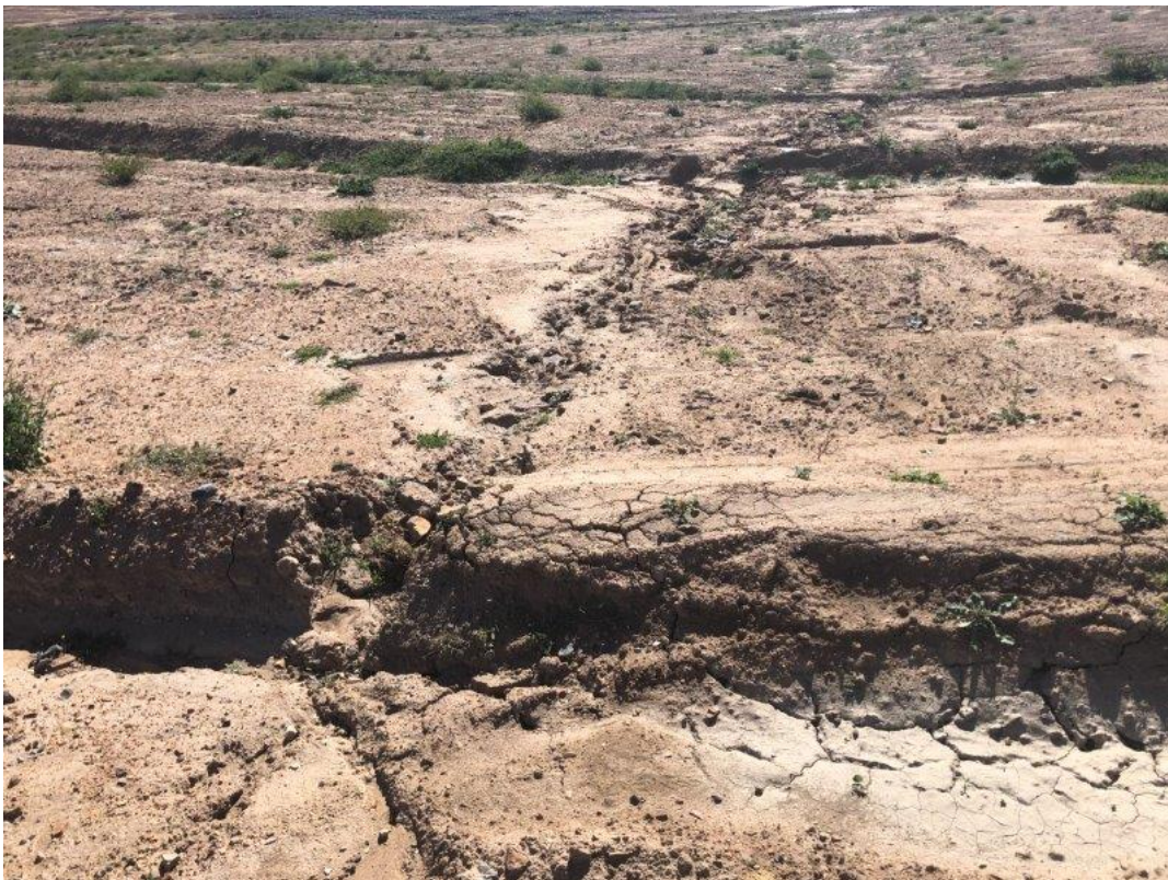
Plate 28 – Example of poor construction of graded bank leading to sedimentation and bank failure.
