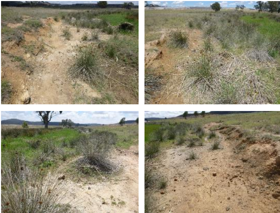
Figure B- 51: CCK2 site photos clockwise from top left: 2017 upstream, 2018 upstream. 2018 downstream, 2017 downstream
