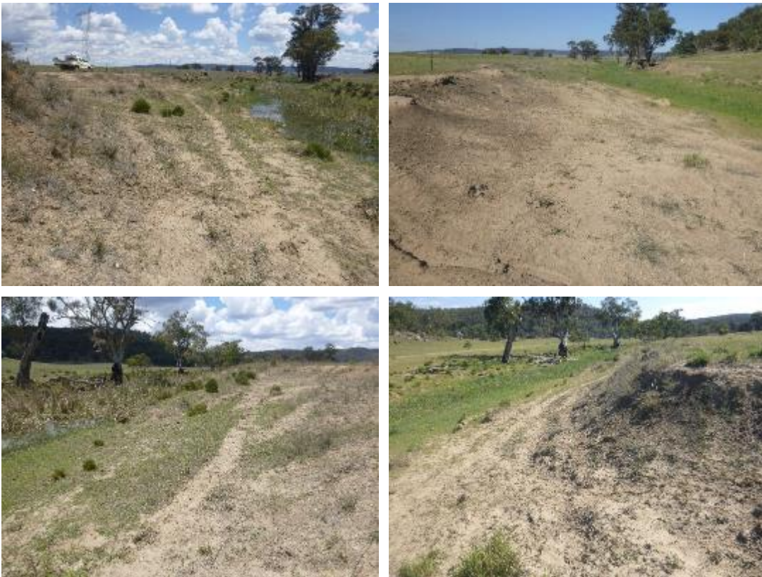
Figure B- 37: WcK37 site photos clockwise from top left: 2017 upstream, 2018 upstream. 2018 downstream, 2017 downstream
