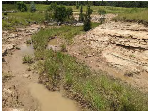
NWCD – Stage 3 near Div 8 – some rock bank erosion (2022)
