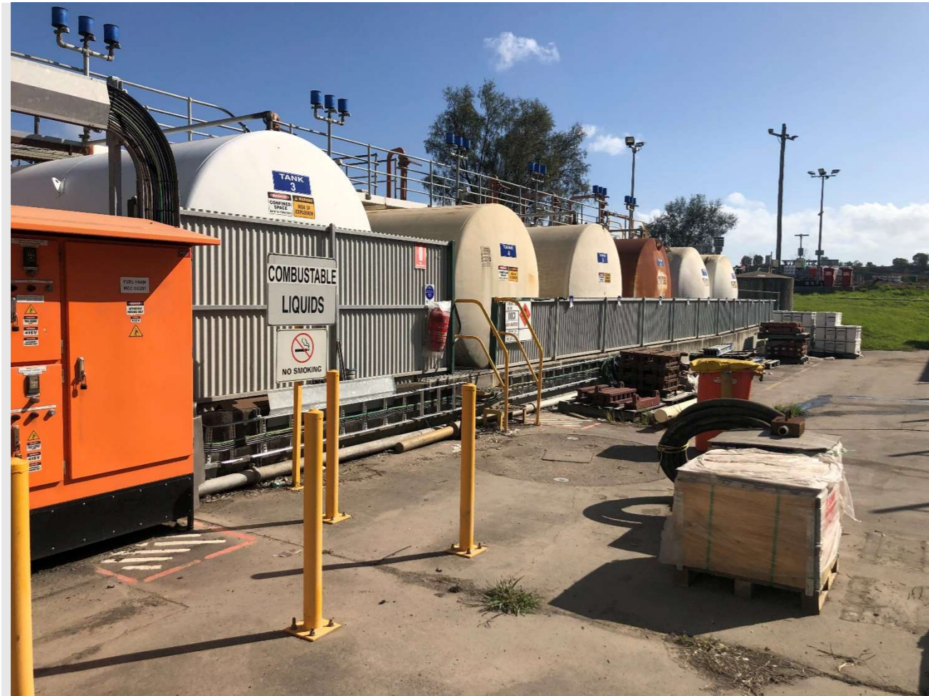
Plate 1 Bunded, above ground storage tanks near the workshop building
