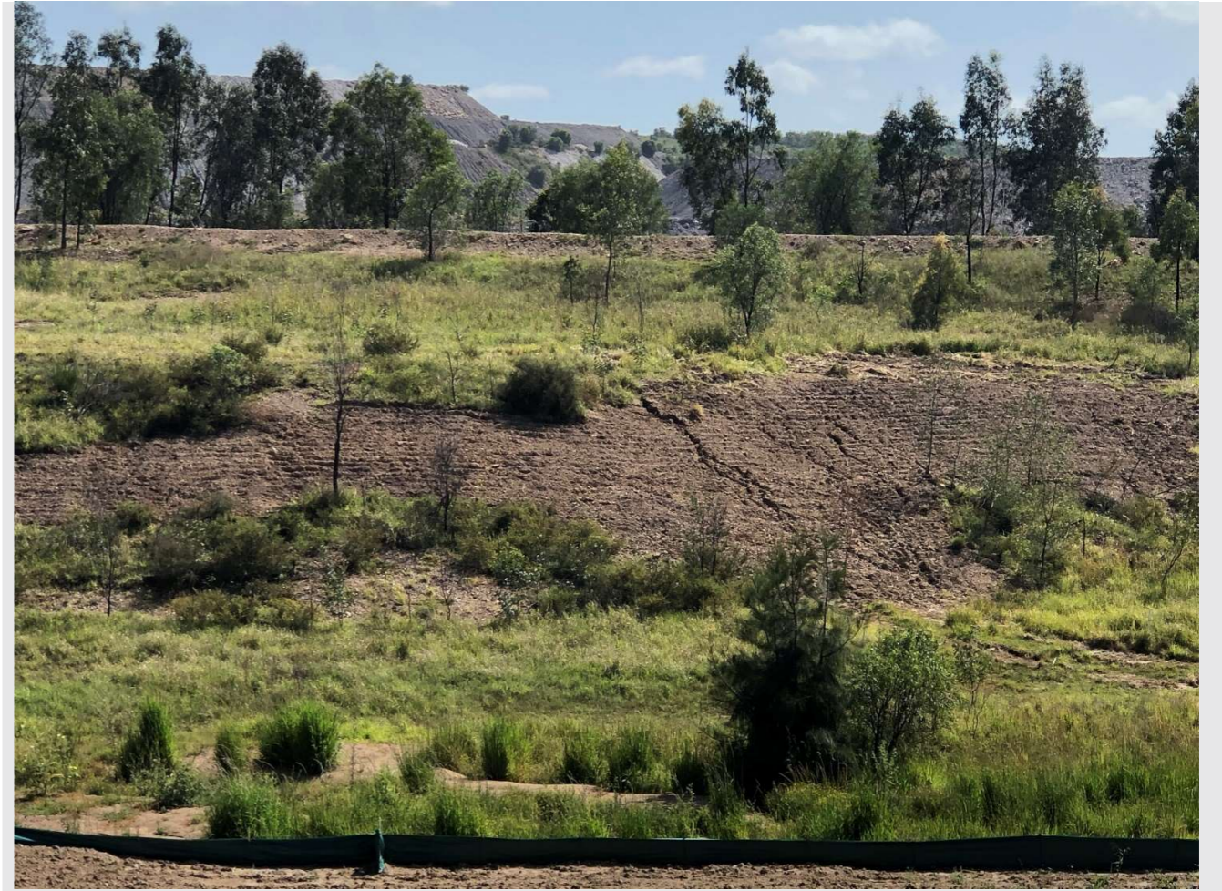
Plate 10 Rehabilitation works currently underway near the North Wambo Creek Diversion to repair subsidence cracking
