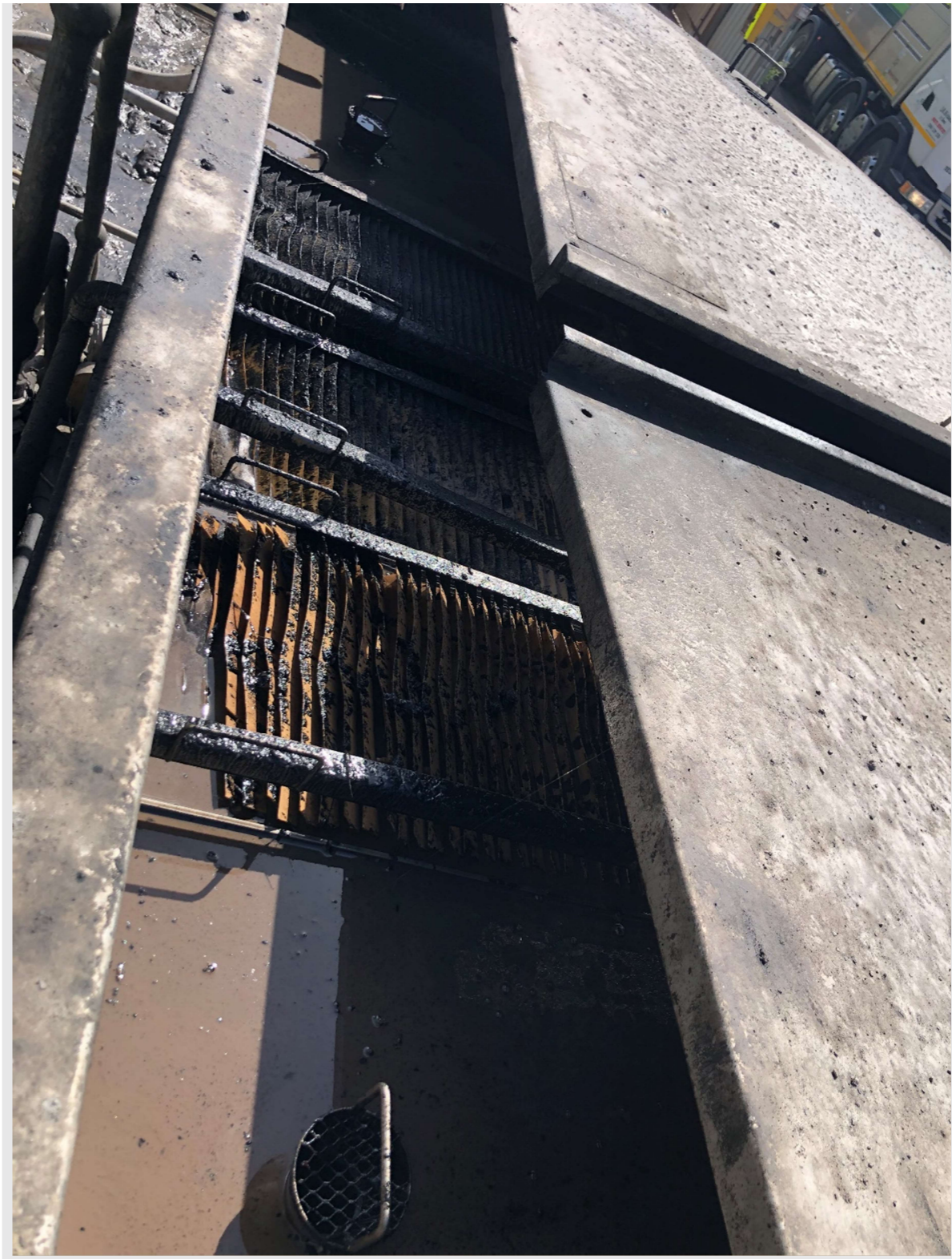
Plate 6 Oil water separator system, serviced by J.R Richards
