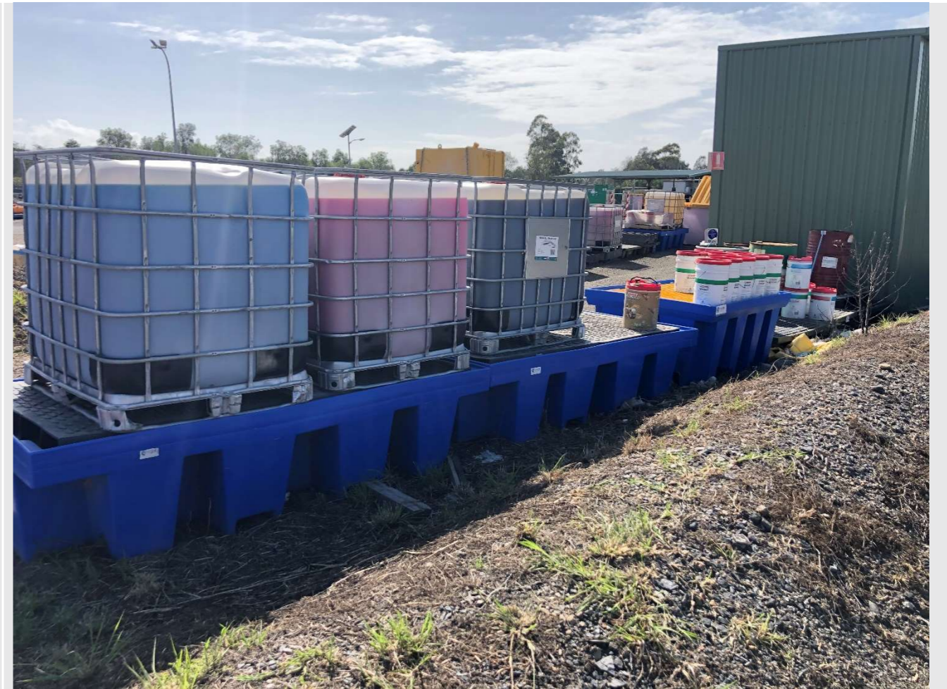
Plate 2 Bunded fuel storage in vicinity of the workshop area
