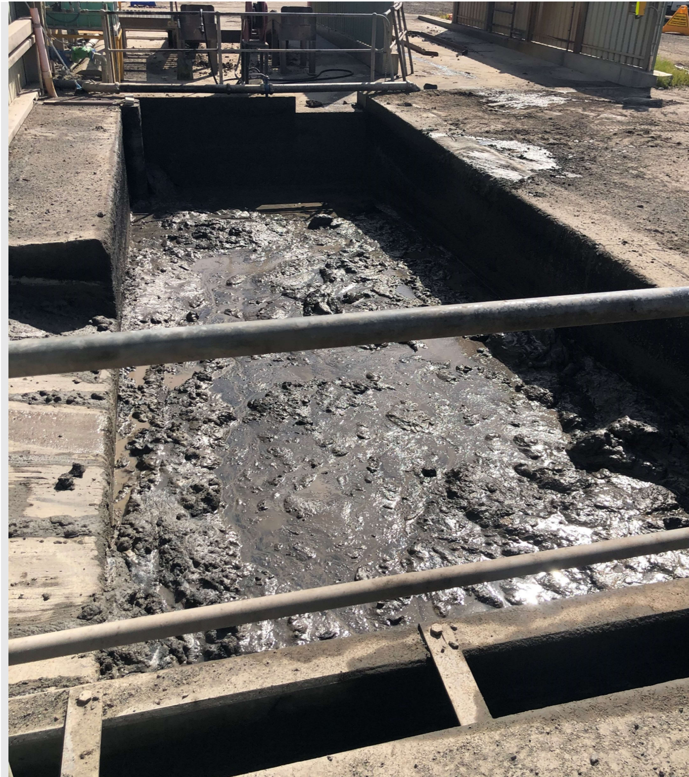
Plate 5 Oil water separator system, serviced by J.R Richards
