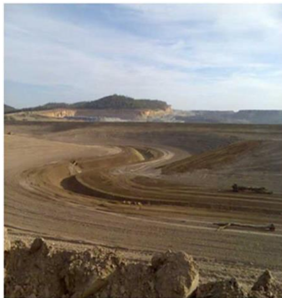
Plate 15: Construction stage of the North Wambo Creek diversion prior to completion in 2008 (Daracon, 2016)
