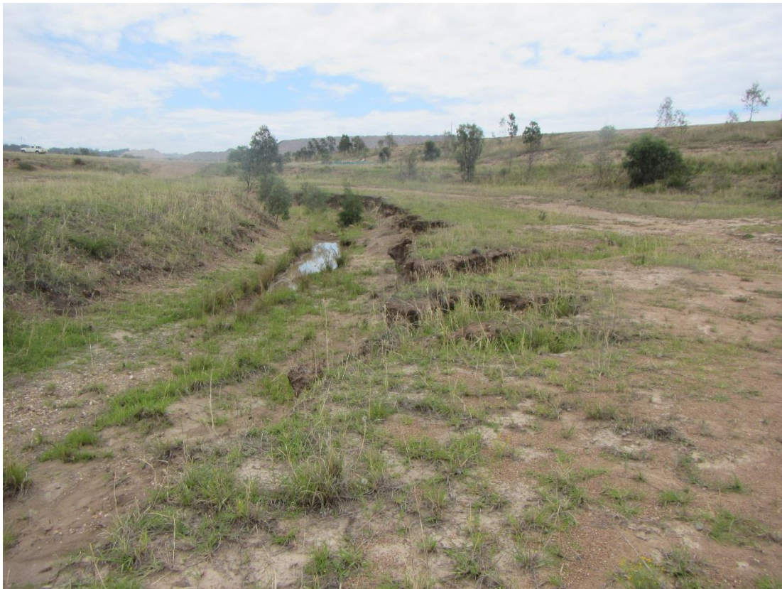
Figure 2-7. Section of NWCD Stage 2 near Div 5 already undergoing erosional adjustment that will be subject to increased erosion risk from LW 11-16 subsidence
