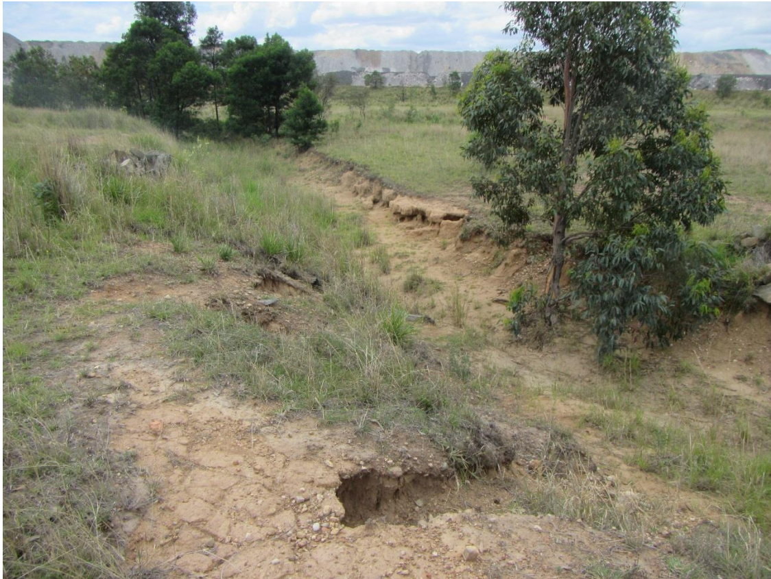
Figure 2-6. Minor overland flow and bank erosion in dispersive soils, mid stage 2 NWCD near Div3
