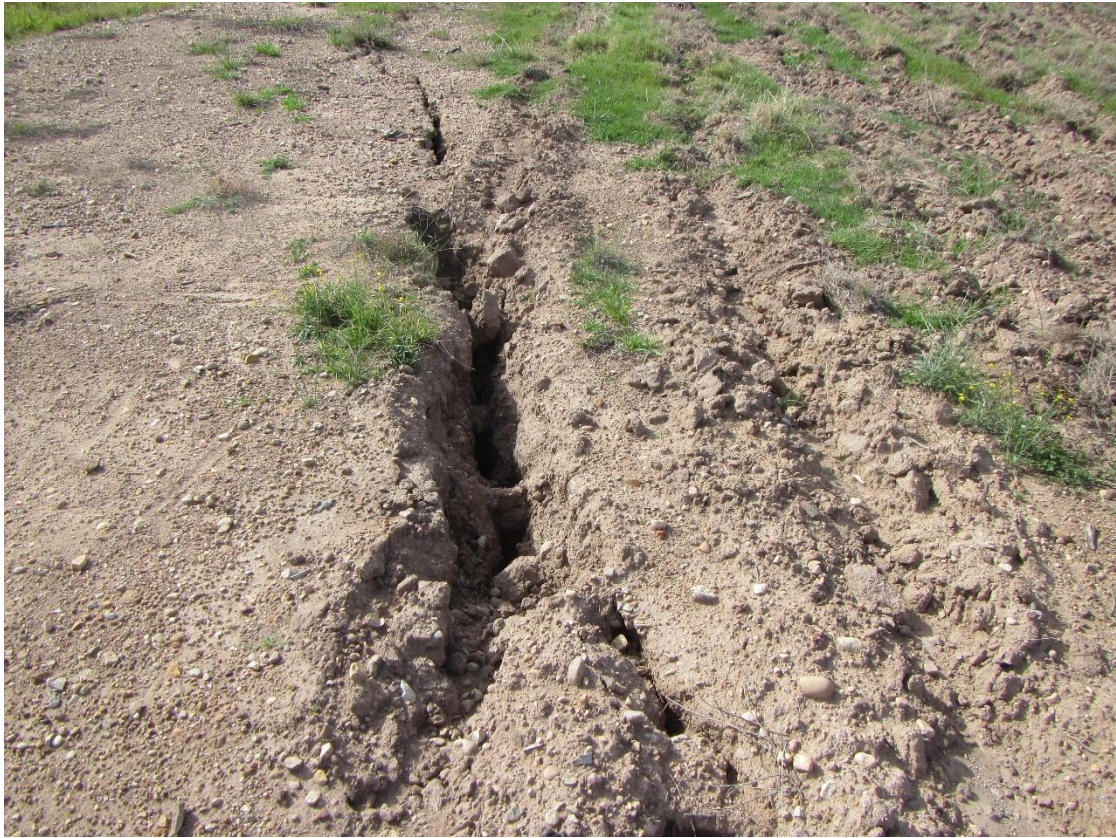
Figure 3-1 - Cracking at surface over LW13/14
