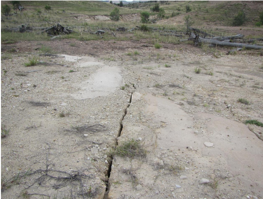
Figure 2-11. Compression buckle cracks at 1-2m spacing through the sandstone in NWCD near Div8 over LW 13/14
