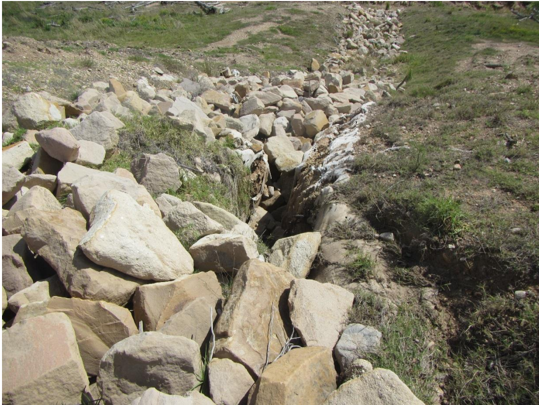
Figure 2-15. Tunnel erosion undermining one of the overland flow entry structures that requires management
