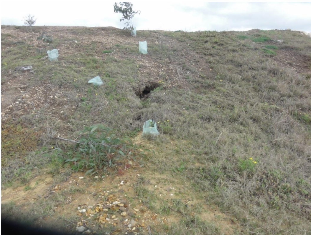
Figure 2-14. Tunnel erosion associated with overland flow management in Stage 3 NWCD is the subject of a management program by Wambo Coal
