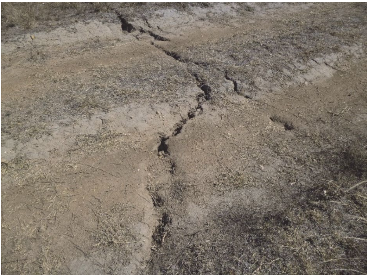
Figure 3-4. Surface Cracking along the Access Tracks above LW17
