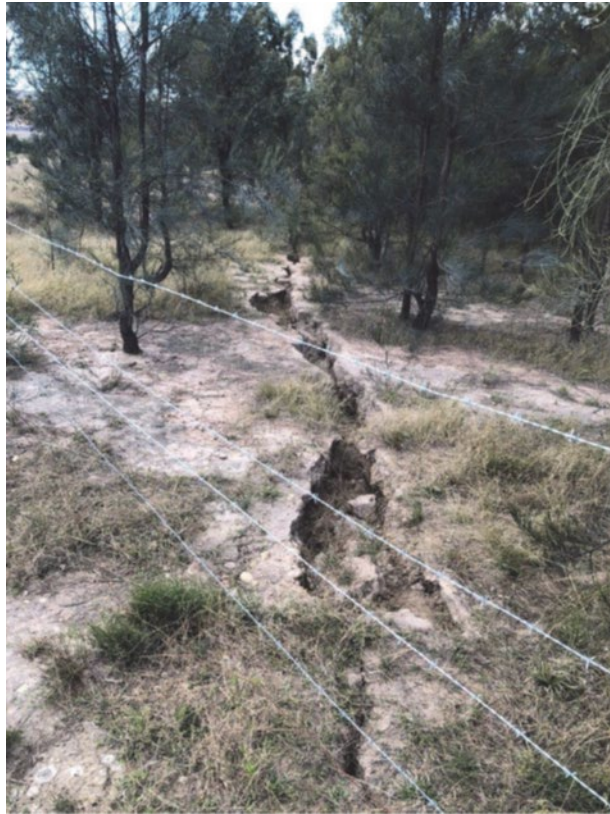
Figure 3-7. Surface cracking near Dam d07 adjacent to the main gate of LW20
