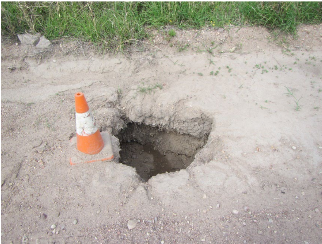
Figure 3-8. Tunnelling over LW12/15 on track adjacent NWCD associated with subsidence crack
