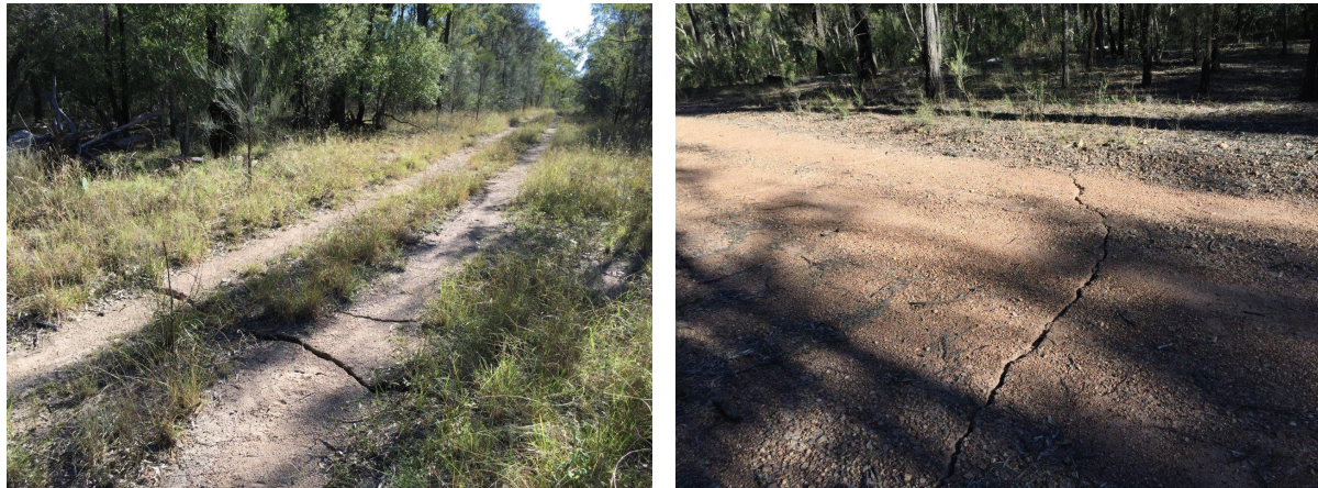
Fig. 4.9 Cracking along the access tracks above the central part of WYLLW13 (Source: WCPL)
