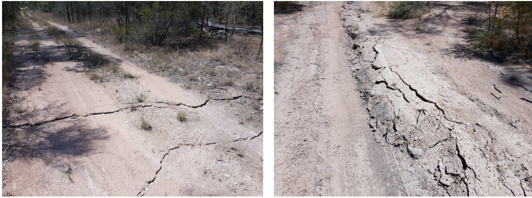
Fig. 4.8 Cracking and compression heaving along the tracks above WYLLW12 (Source: WCPL)
