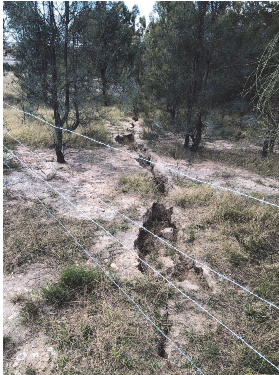
Fig. 4.13 Surface cracking near Dam d07 adjacent to the maingate of WYLW20 (Source: WCPL)
