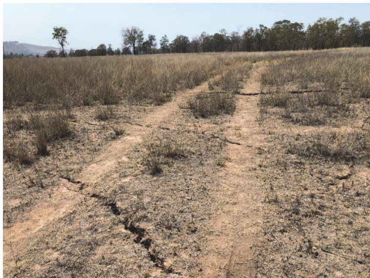
Fig. 4.9 Surface cracking near the finishing end of WYLW18 (Source: WCPL)
