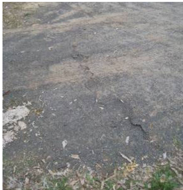
Fig. 4.14 Surface Compression Buckling Observed in a Pavement
