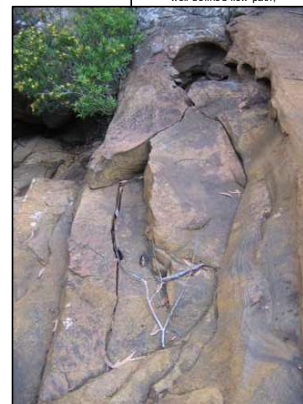
ETZ-10 Cracking at step down in sandstone
