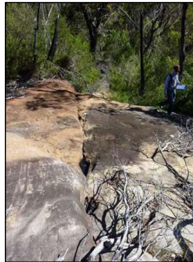
TB069-6 Joint with water
