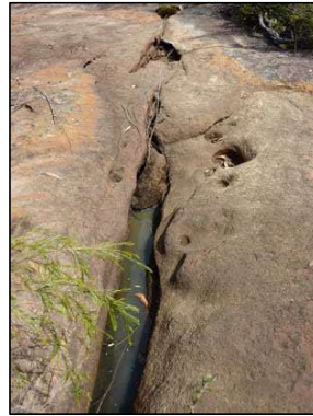
TB120-3 Joint with water
