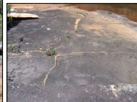
G1-14 Crack perpendicular to joint
